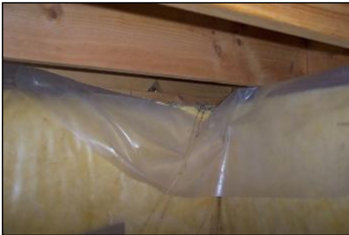
Vapor Barrier Compromised - Right Rear
