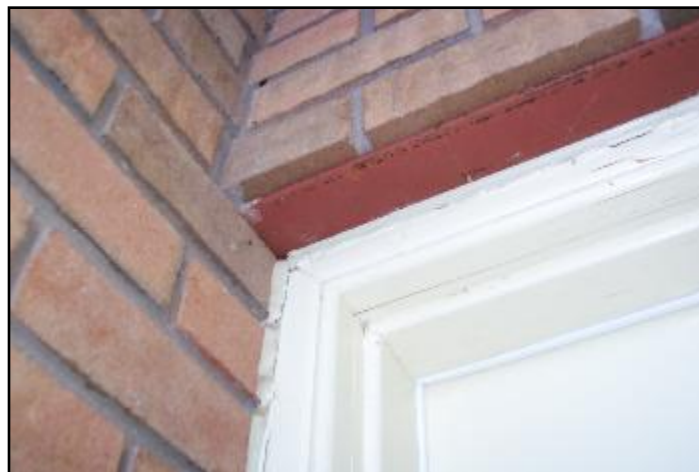
Surface Rust on Underside of Lintel
