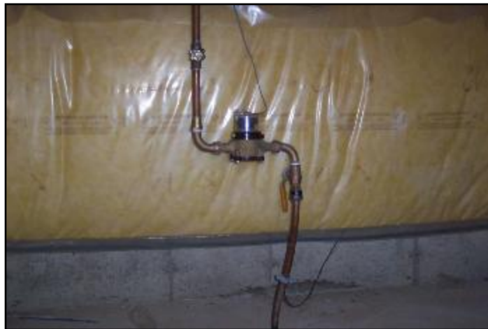
Water Meter and Shut Off Location
