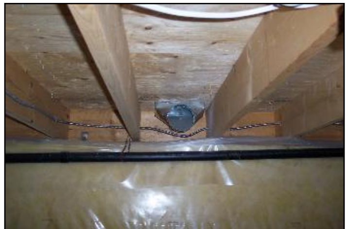
Duct Disconnected at Register
