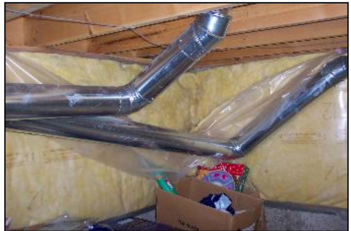
Vapor Barrier Compromised - Front Middle
