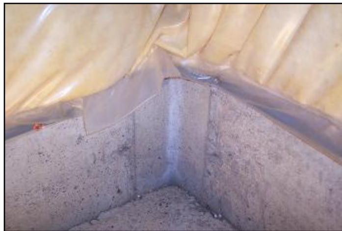
Efflorescence at Front Left Corner
