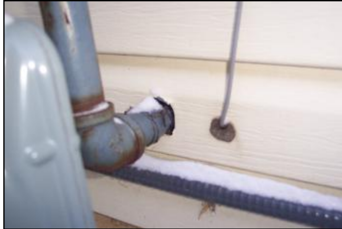
Caulking Required at Gas Line Entry
