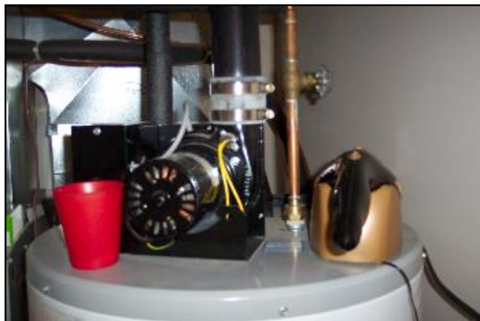
Items Stored on Water Heater
