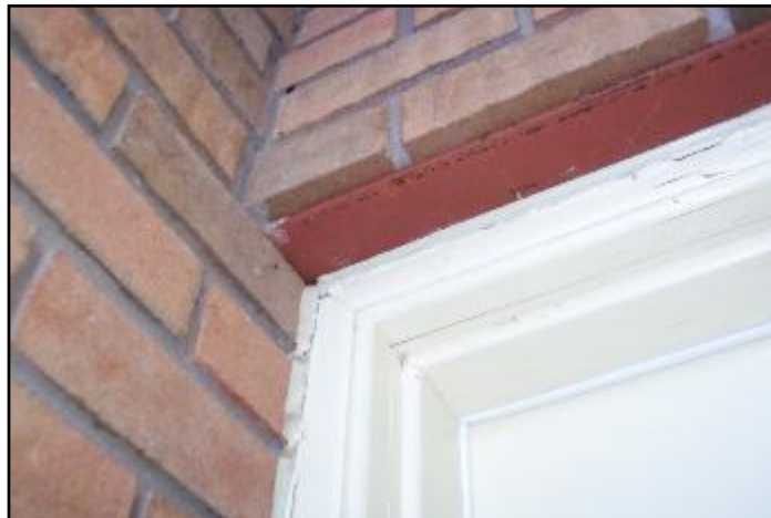
Deteriorated Caulking and Minor Rust
