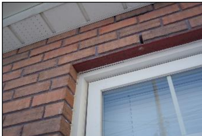
Surface Rust on Lintel and Caulking Required
