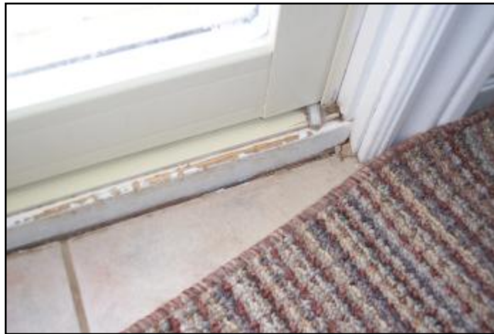
Grout Missing at Sliding Door Entrance
