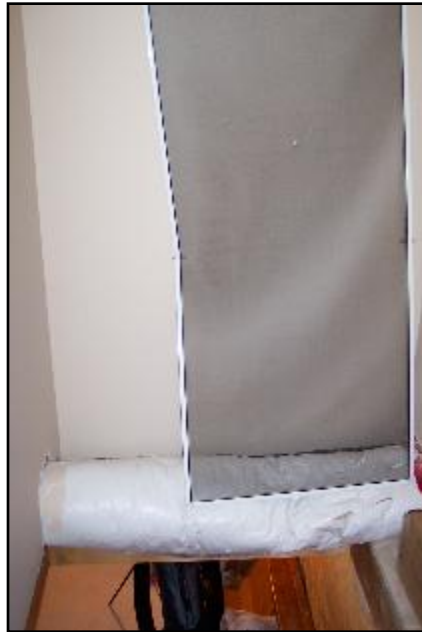
Screen Found at Crawl Space Entrance
