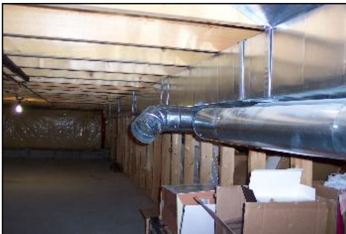
Duct Disconnected at Trunk
