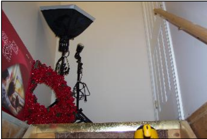
Trip Hazard at Top of Crawl Space Stair
