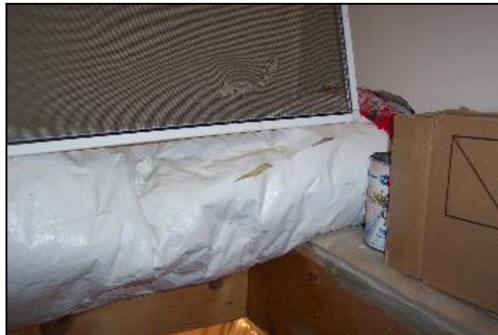
Cuts in Duct Insulation
